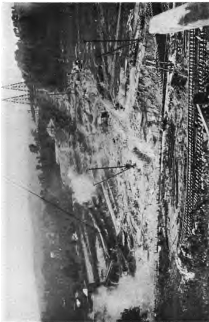
PLATE 183.—Contract 9. Kensico Dam Foundations. Cableway towers for span of 1950 Feet. Excavation mostly removed by steam shovels. Remains of old Kensico Dam at Left.
